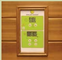
Dual control panels
